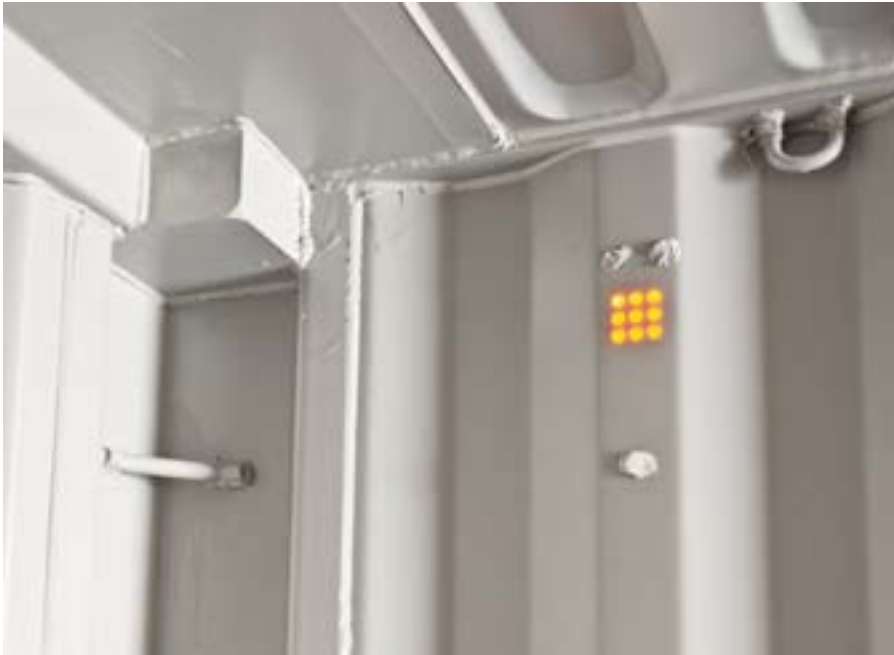
Lashing points in a standard container on the roof edge, at the corner post and small vents for air-pressure equalisation
